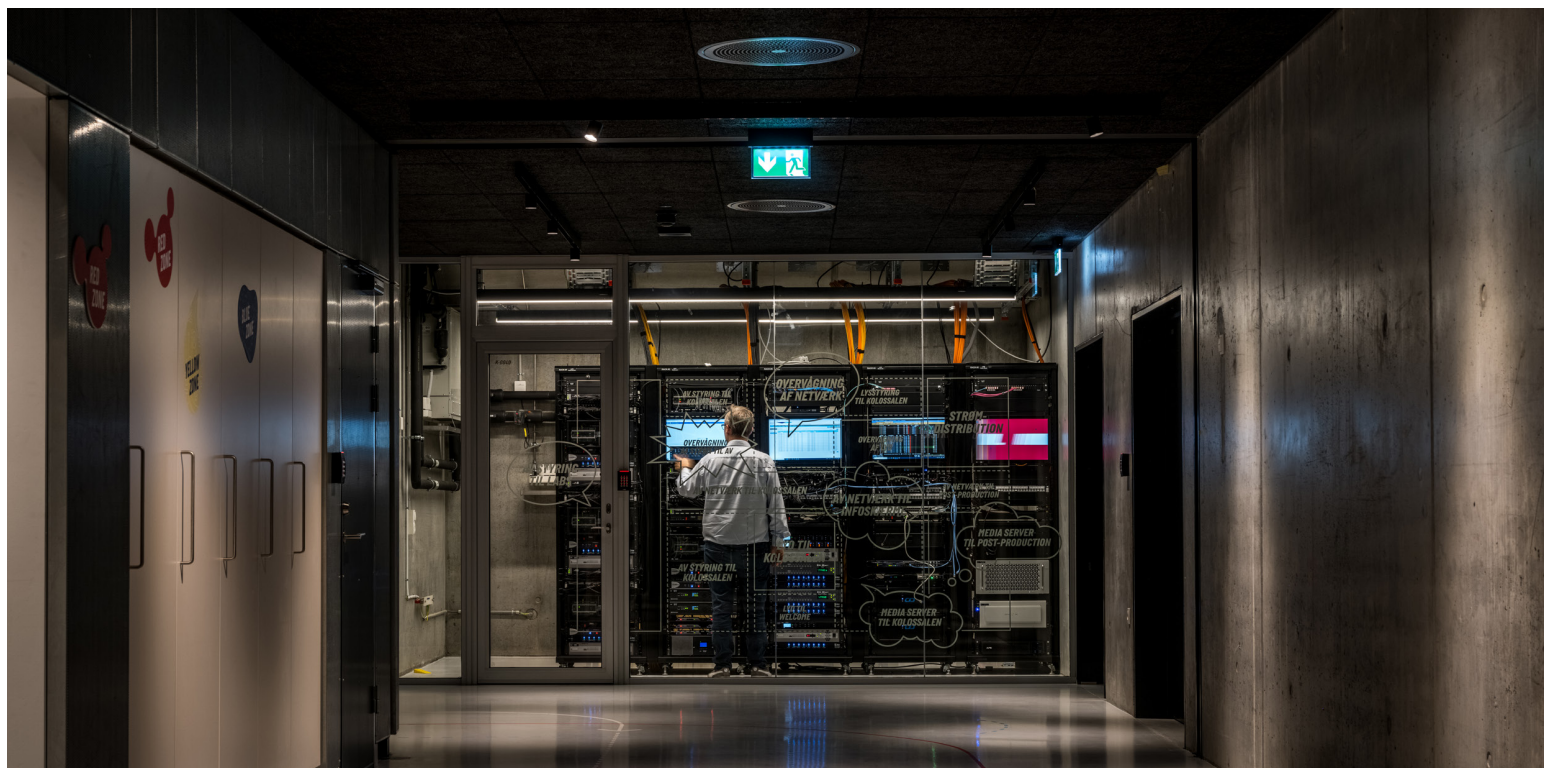
The rack room at LIFE is one of the attractions of the building
